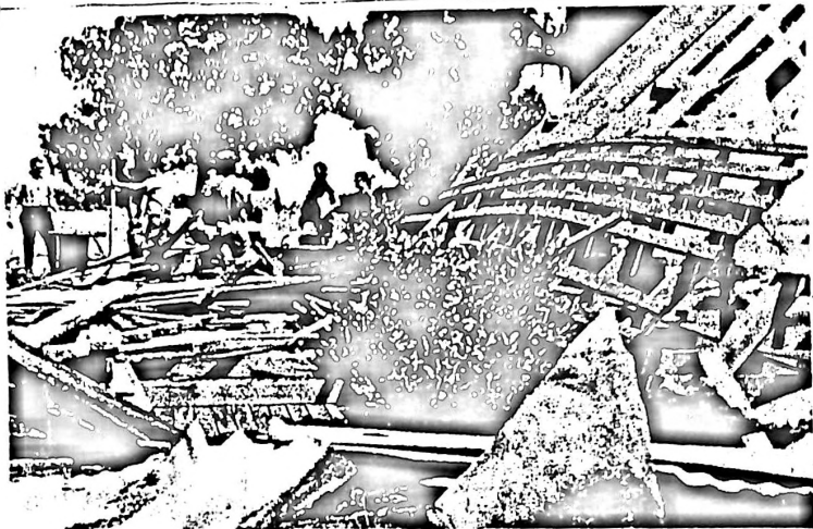
GETTING READY – Looking across the fallen Ozello school building, on School House Island, above picture shows Ozello citizens preparing to install American and Bicentennial flagpoles, prior to starting project to restore the ancient school.
