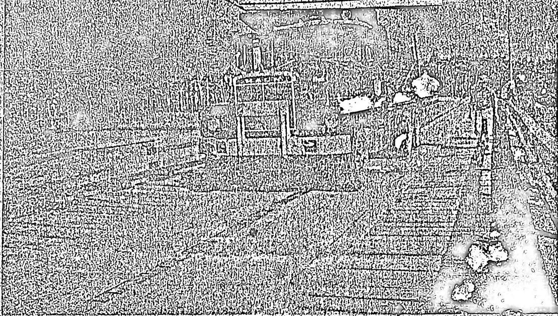
BRIDGE EXAMINATION — Citrus County Commissioner Catherine Rooks and Road Superintendent Myron Townsend, examining a piling under the Black Creek bridge near Ozello Wednesday after repairs were made to the wooden structure. The bridge was tested by driving an 11-ton Mack truck over the structure prior to weight limits being increased to 10 tons.
